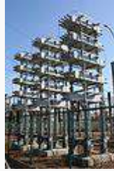
75MVAR substation capacitor bank at 150kV
